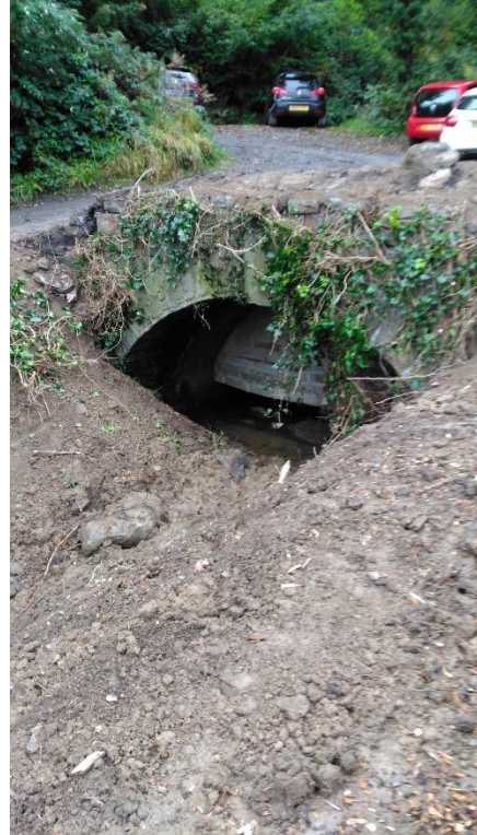
Damaged communal air raid shelter, Ynystawe
